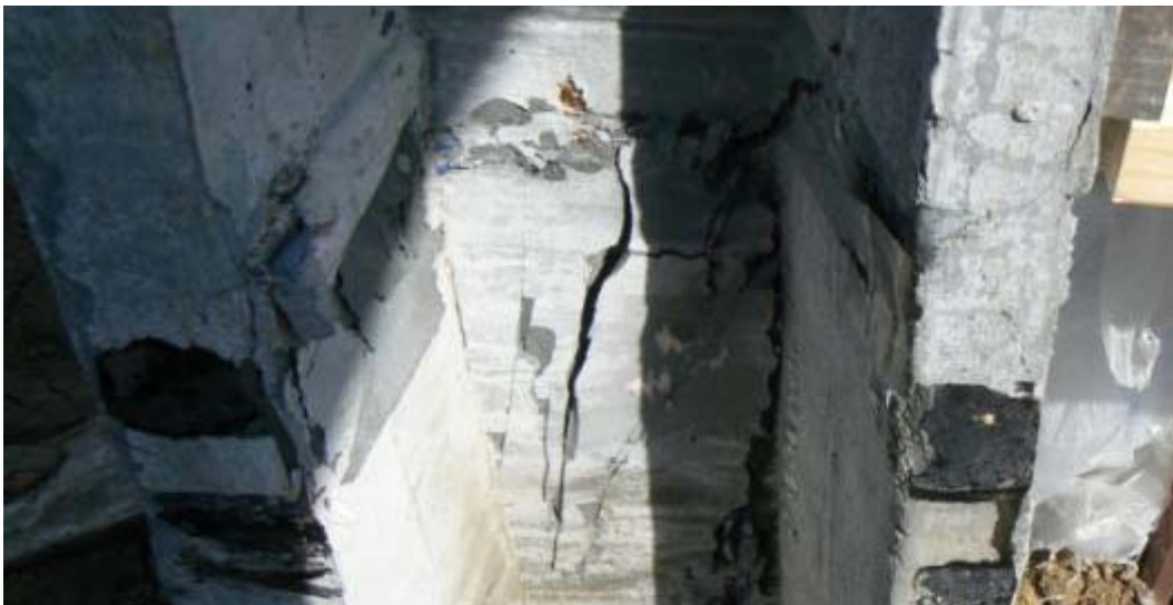
Figure 5.43. Initial shear cracking in web of UHPC pile P1 at a lateral load of 22.8 kip (101.3 kN)
