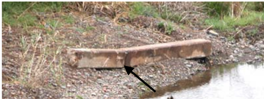
Figure 1.1. Precast, prestressed concrete pile cracked during driving (RTA NSW 2005)
