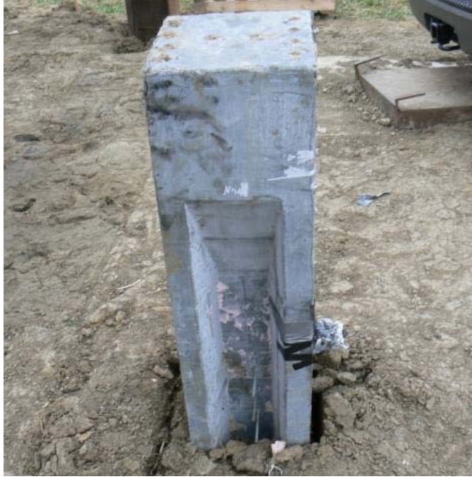
Figure 5.36. Condition of pile P2 at the end of the lateral load test
