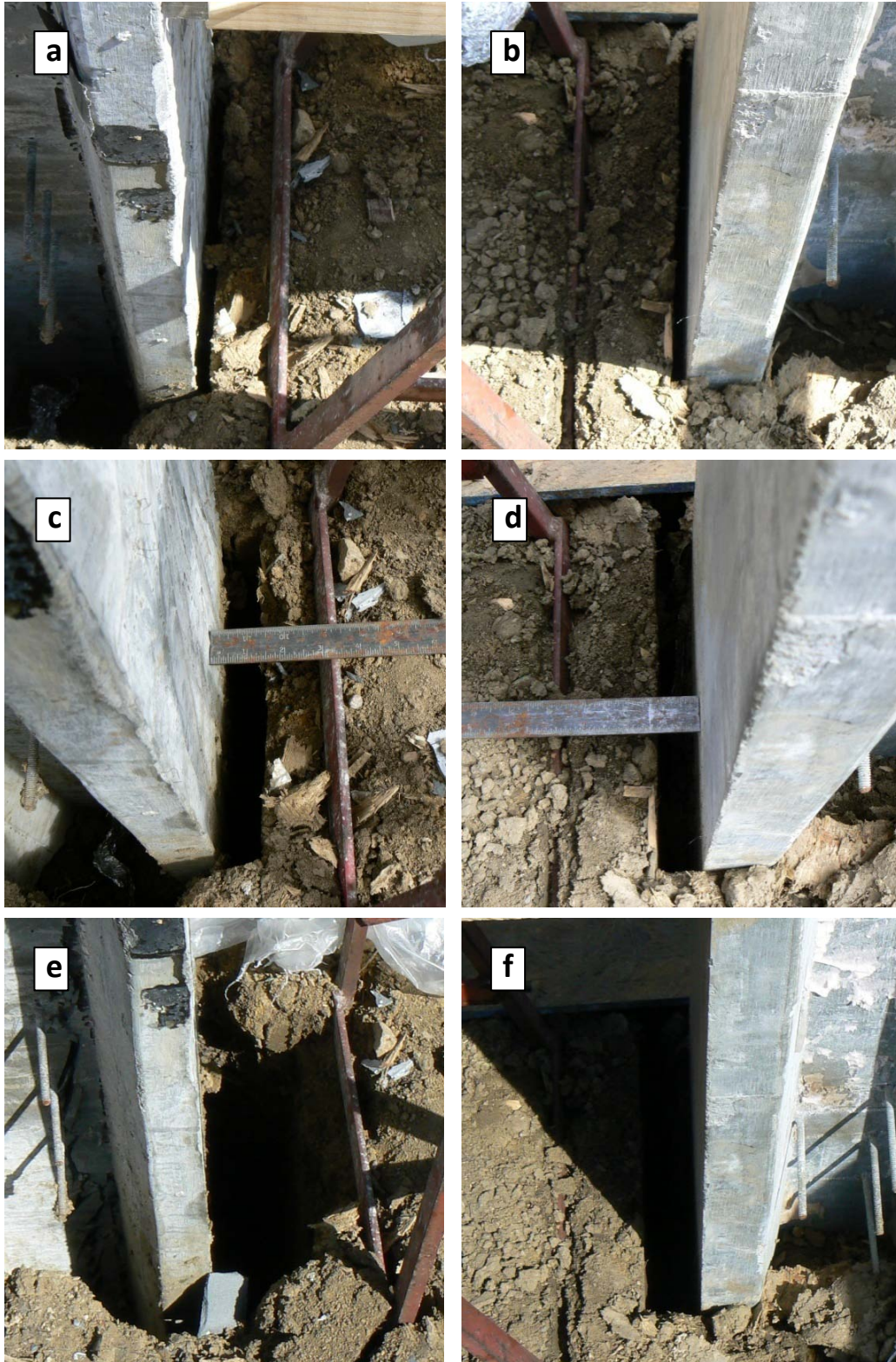
Figure 5.35. Soil gaps due to lateral pile movement next to a) P1 and b) P2 early in the test, c) P1 and d) P2 midway through the test, and e) P1 and f) P2 after the shear failure of pile P1
