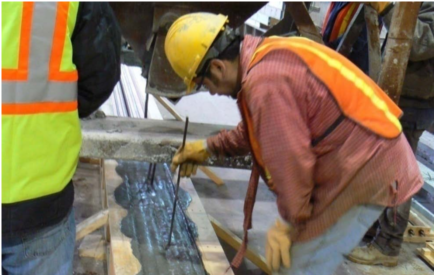
Figure 4.24. “Rodding” through the web of UHPC to eliminate formation of possible air pockets
