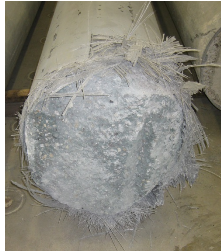
Figure 22: Cut at Failure of Pile G-4FB
