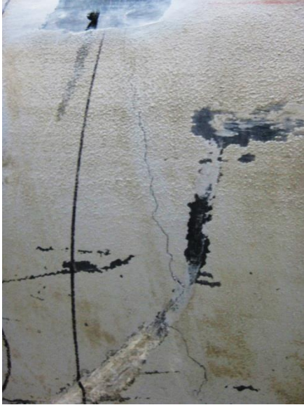
Figure 37: Cracks in Constant Moment Region
