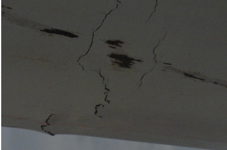
Figure 30: Cracks Due to Cyclic Loading
