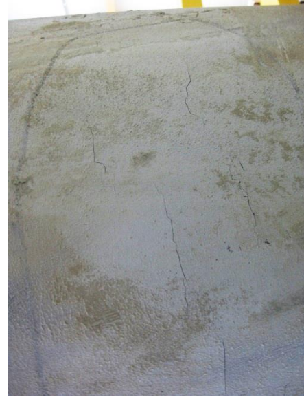
Figure 38: Cracks Out of Constant Moment Region
