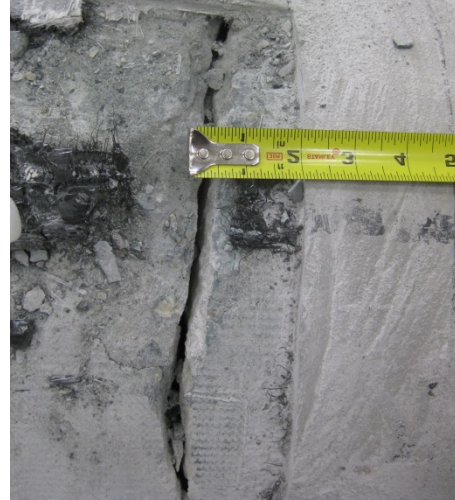
Figure 28: Crack in Pile A's Concrete at Compression Wrinkle
