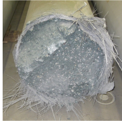
Figure 26: Cut at Failure of Pile A-4FB
