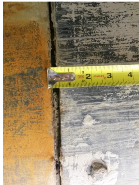
Figure 29: Loss of Composite Action in Pile A
