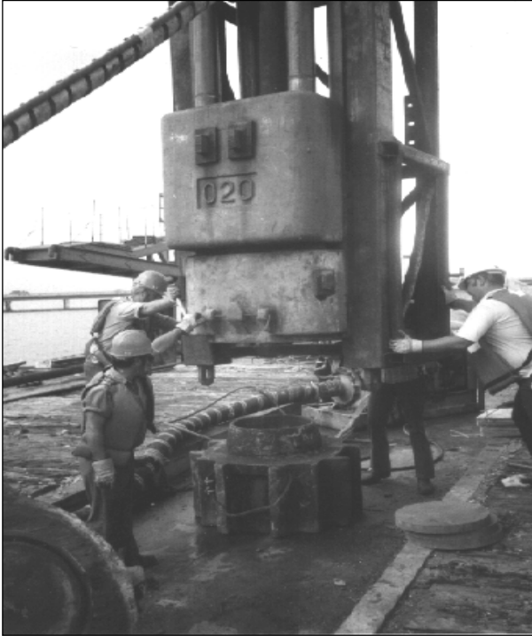
Figure 23.2 Hammer Cushion Check
