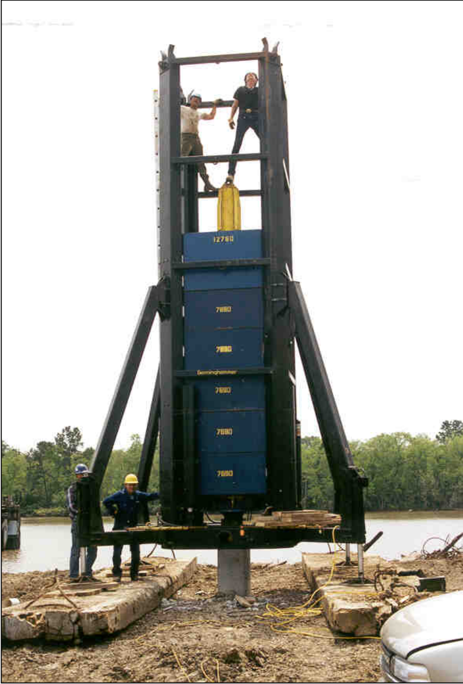
Figure 20.2. 4,400 kN (1000 kip) hydraulic catch device on prestressed concrete pile. (courtesy of Applied Foundation Testing)
