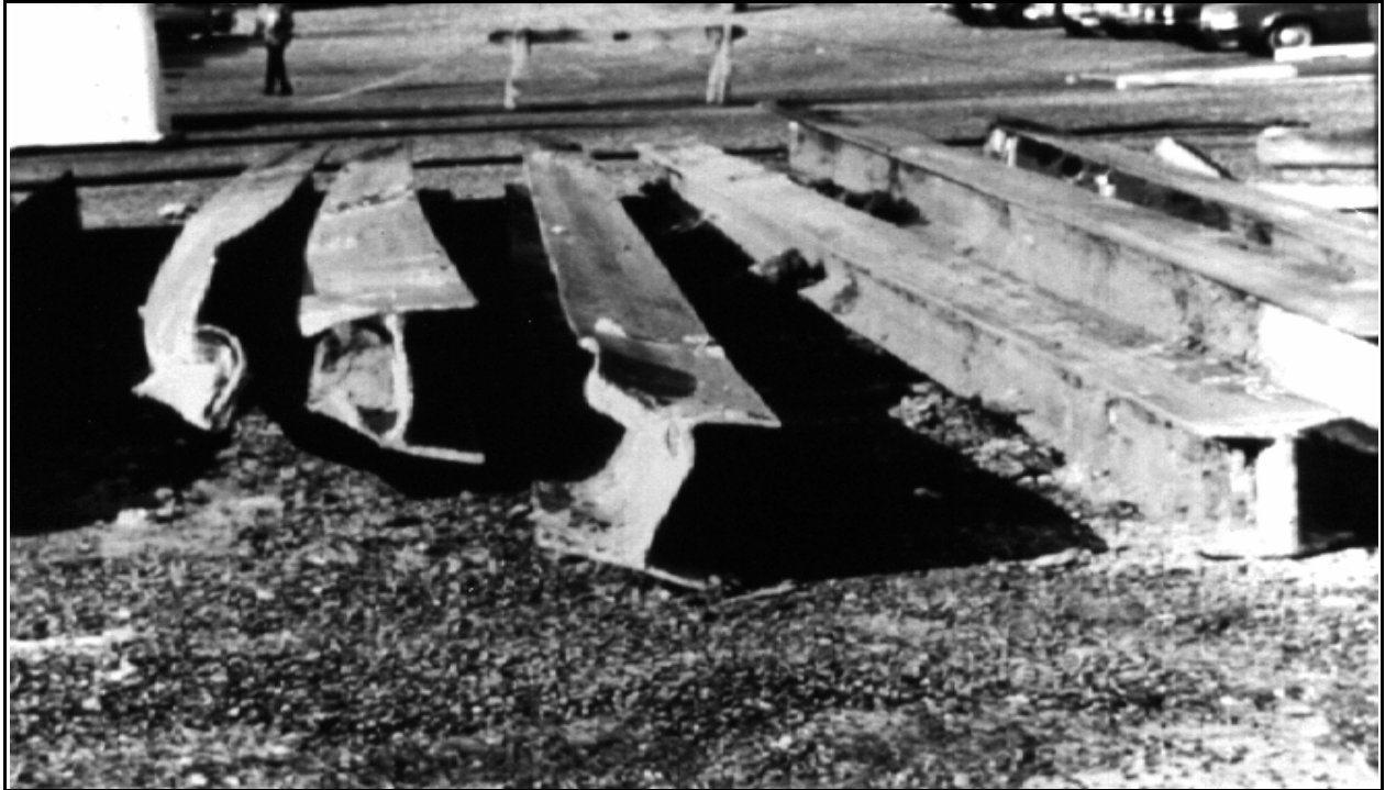
Figure 22.4 Damaged H-piles without Pile Toe Protection
