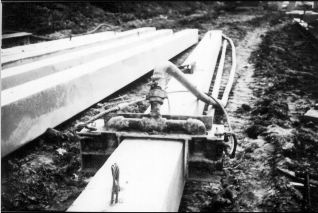
Figure 21.34 Dual Jet System Mounted on a Concrete Pile (courtesy of Florida DOT)
