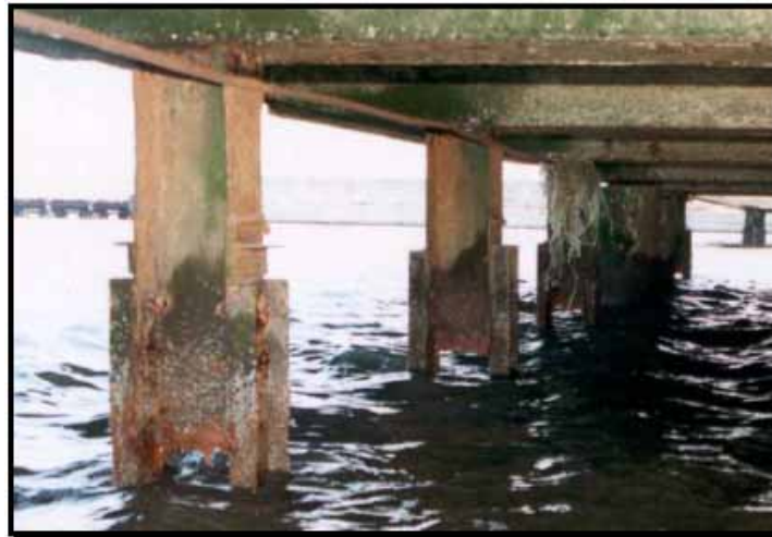
Figure 2. Photo. Complete corrosion of steel H piles supporting a harbor pier (recently installed retrofit channels are already corroding). (9)
