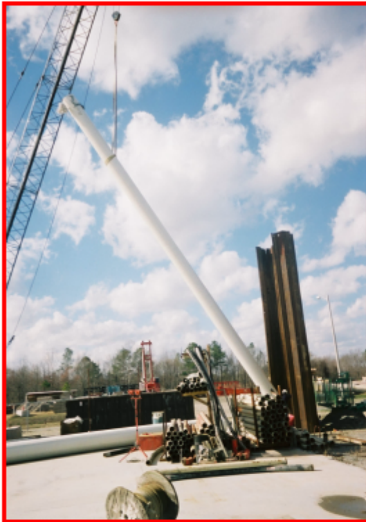
(a) FRP tube with steel cage inside is placed vertically to prepare for concrete filling
