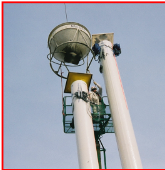
(c) Concrete pouring is controlled by operators located in the adjacent manhole lift
