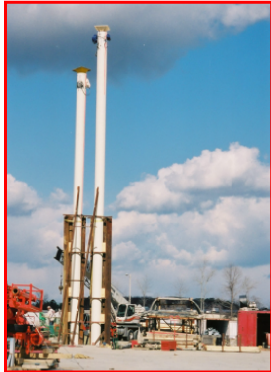
(b) Bracing system used to secure FRP tube and steel cage in a vertical position
