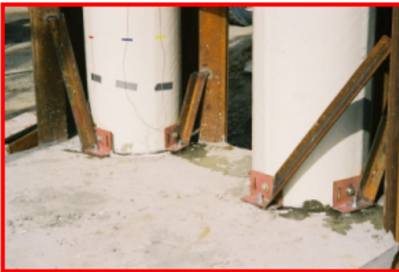
(c) The base of the FRP tubes is bolted to a concrete slab
