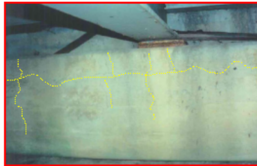
(c) Map cracking in beams
