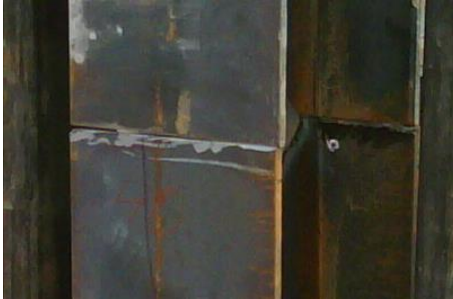
Figure 16-38 H-pile splice preparation without adequate root opening or bevel.
