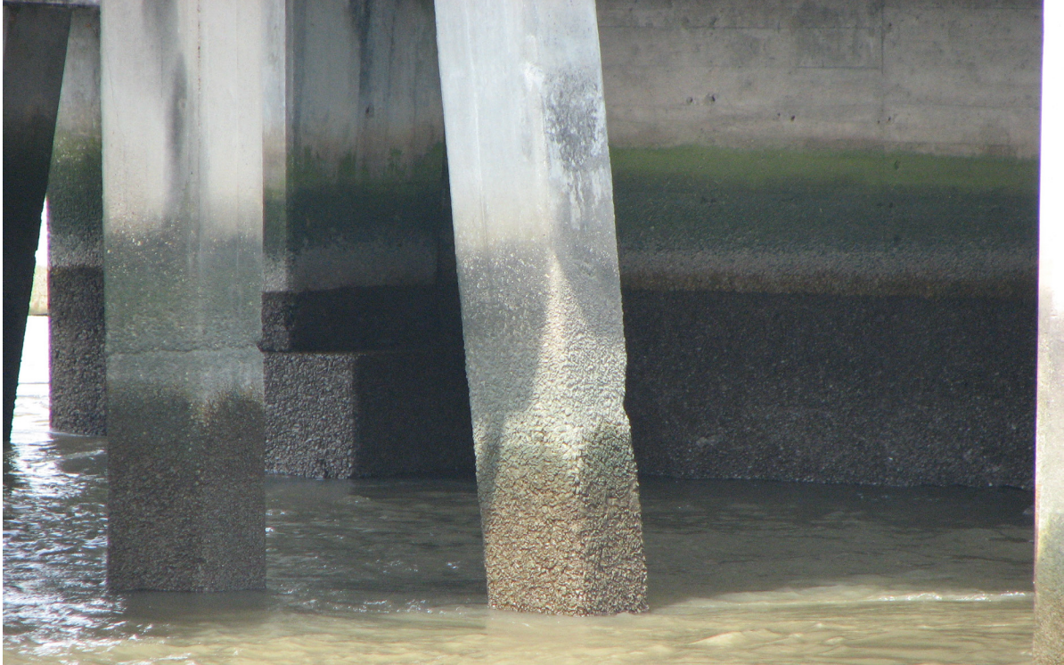
Figure 3-12 Concrete surface abrasion and deterioration in tidal zone (courtesy of Moser 2011).
