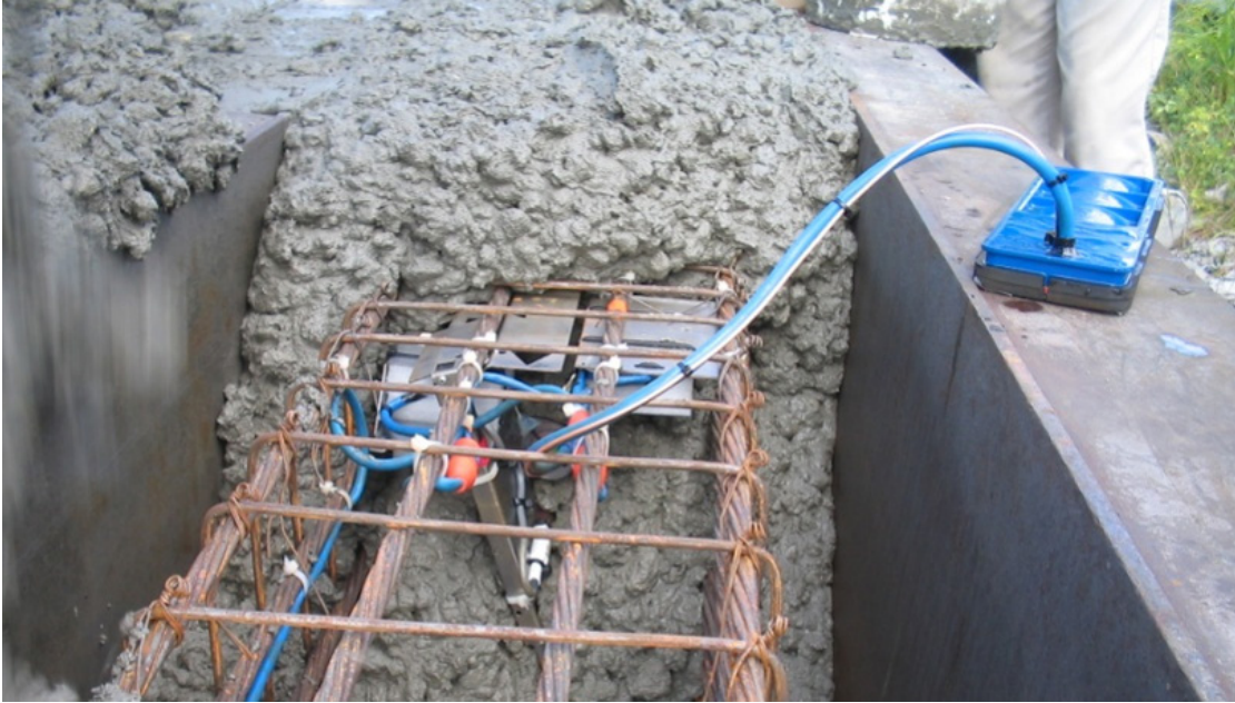
Figure 10-3 Embedded strain gage and accelerometer unit being cast into concrete pile (courtesy Radise International).
