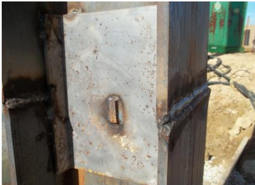
Figure 16-39 Misalignment between pile sections and poor quality weld.
