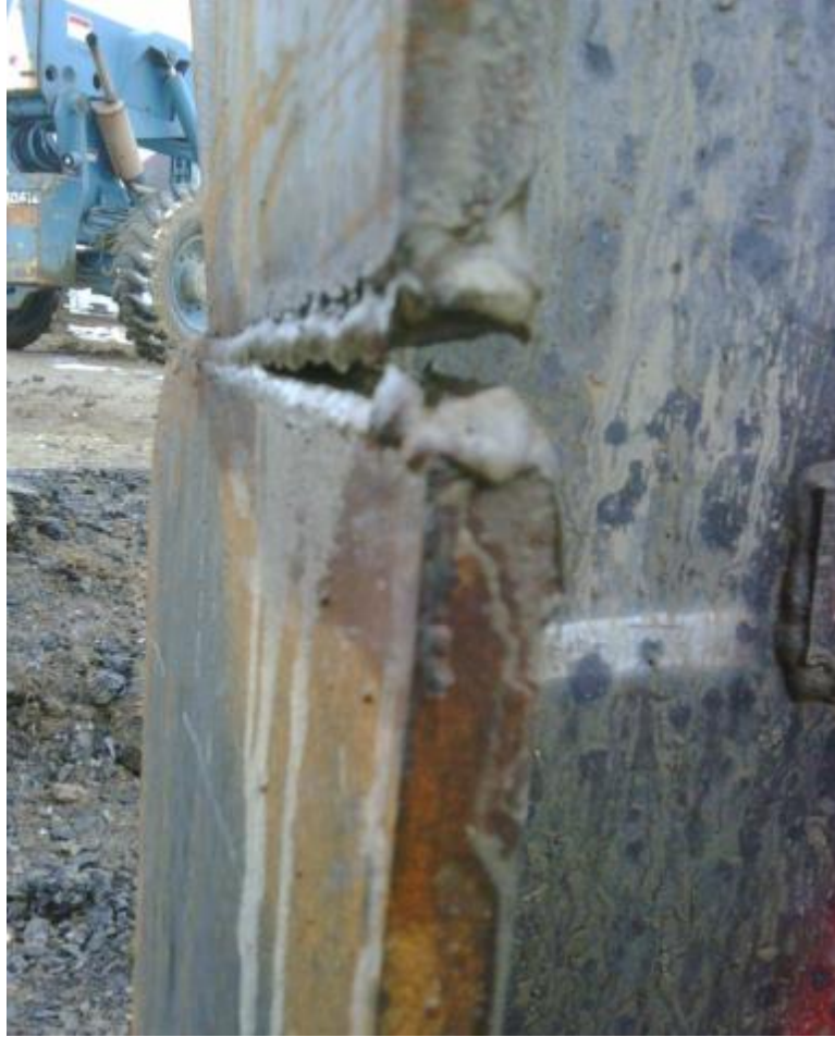
Figure 16-35 Broken weld on H-pile splice.
