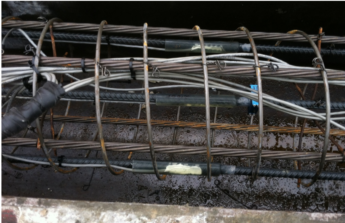
Figure 9-24 Electrical resistance strain gage on sister bars in concrete pile casting bed.
