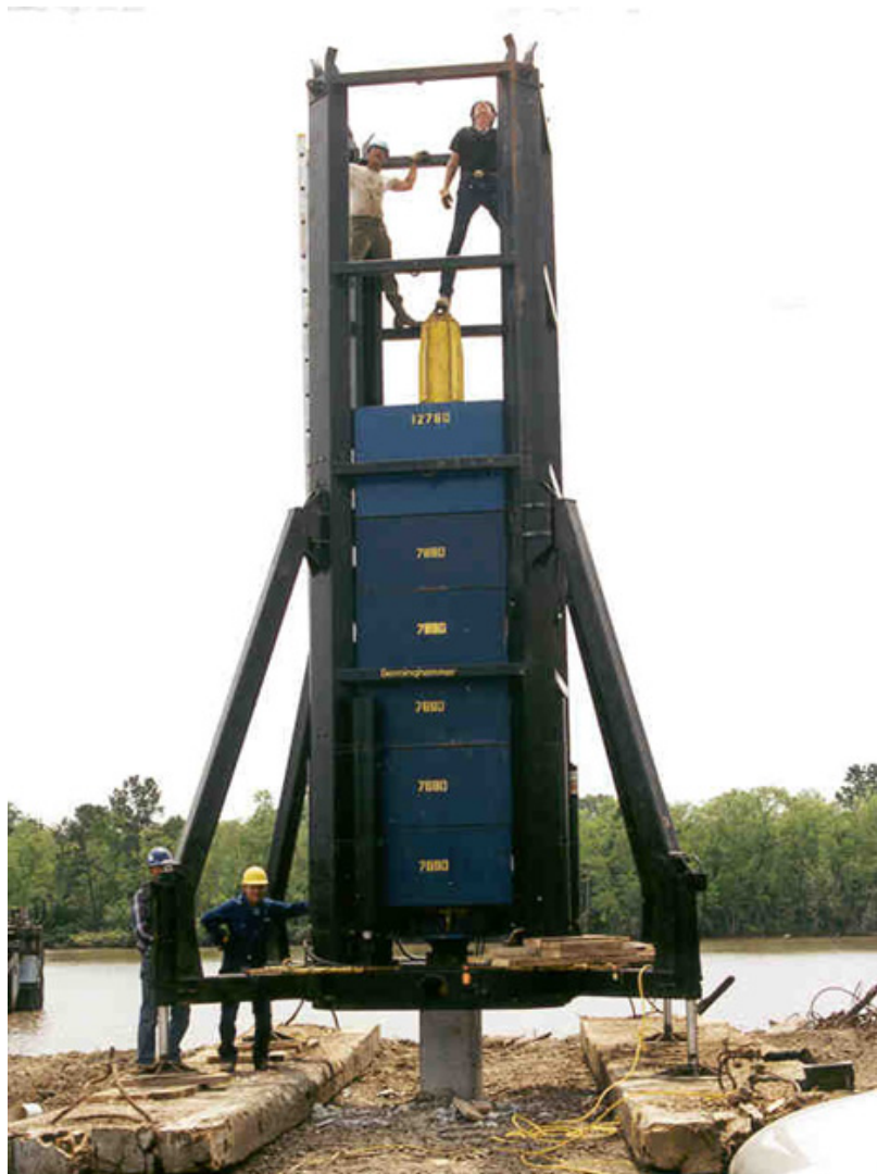
Figure 11-3 1000 kip hydraulic catch device on prestressed concrete pile (courtesy of Applied Foundation Testing).
