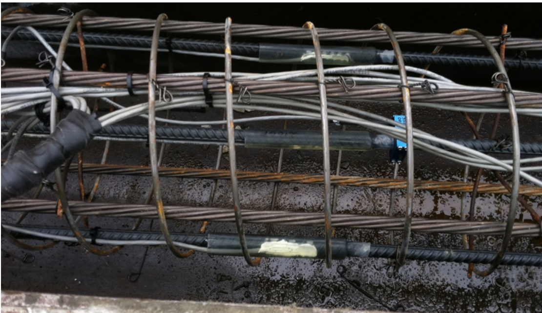
Figure 10-4 Embedded resistance strain gage and accelerometer mounted on sister bar being cast into concrete pile (courtesy of Pile Dynamics, Inc.).
