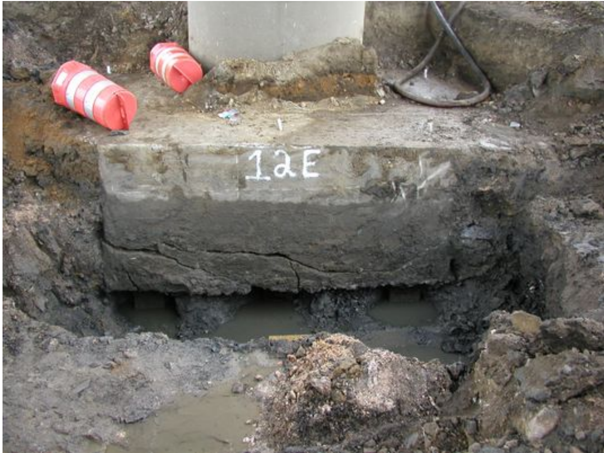
Figure 3-15 Cracked pile cap from lateral soil movements (courtesy DeIDOT).
