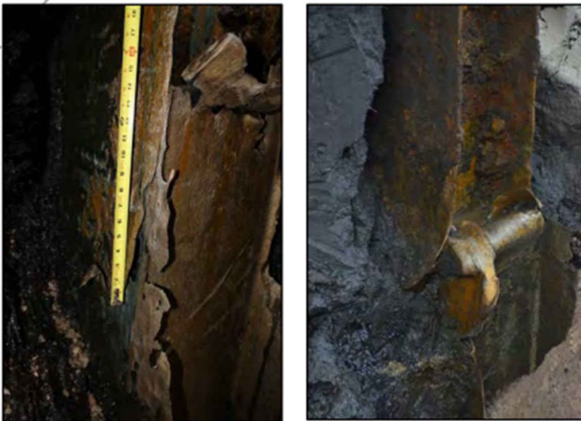
Figure 3-10 Corrosion and resulting buckling of foundation pile (courtesy Wisconsin Department of Transportation).
