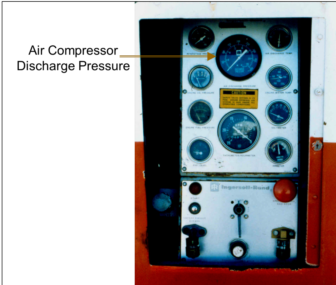
Figure 18-7 Air compressor display panel.
