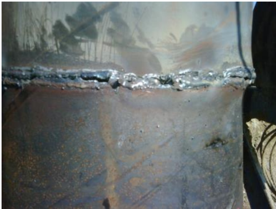
Figure 16-34 Cracked weld on pipe pile splice.
