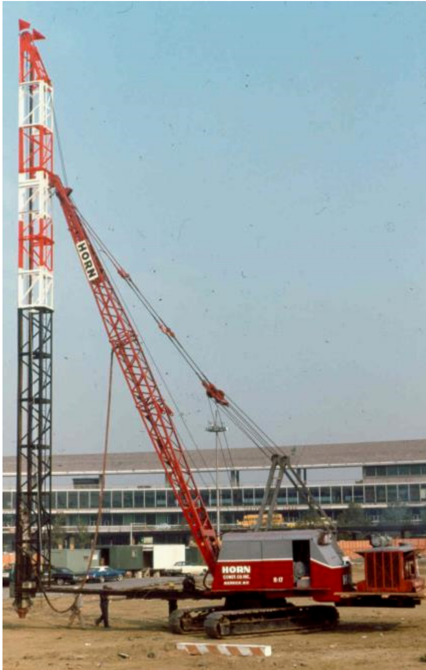
Figure 15-11 Fixed lead system with air compressor mounted as counterweight (courtesy FHWA Demo 66).
