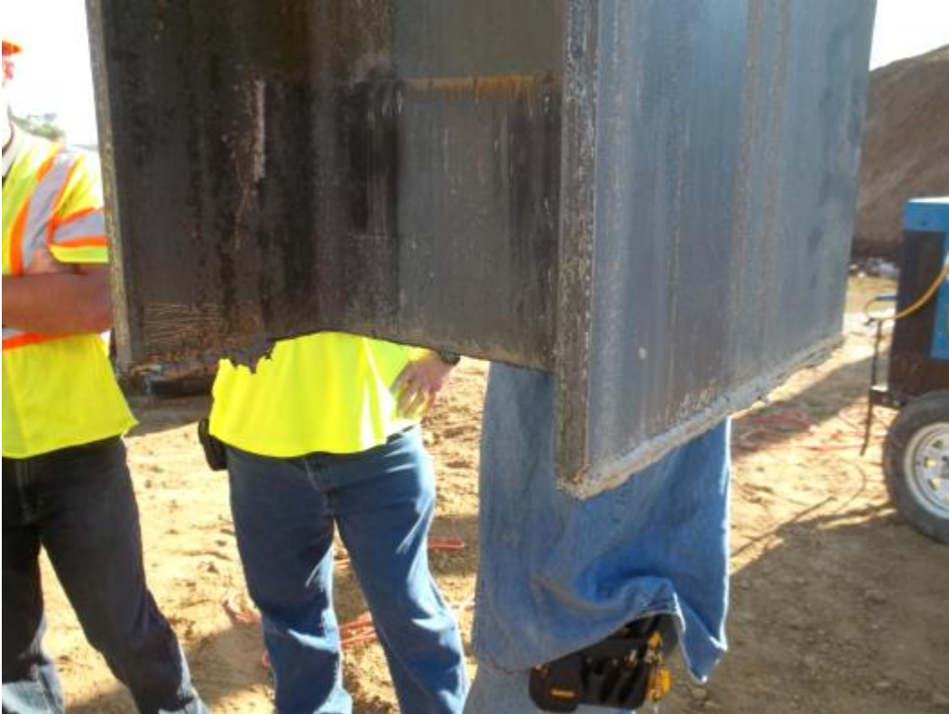
Figure 16-40 Extracted H-pile upper section. Weld cracked during driving and extracted section retrieved without H-pile splicer or lower pile section.
