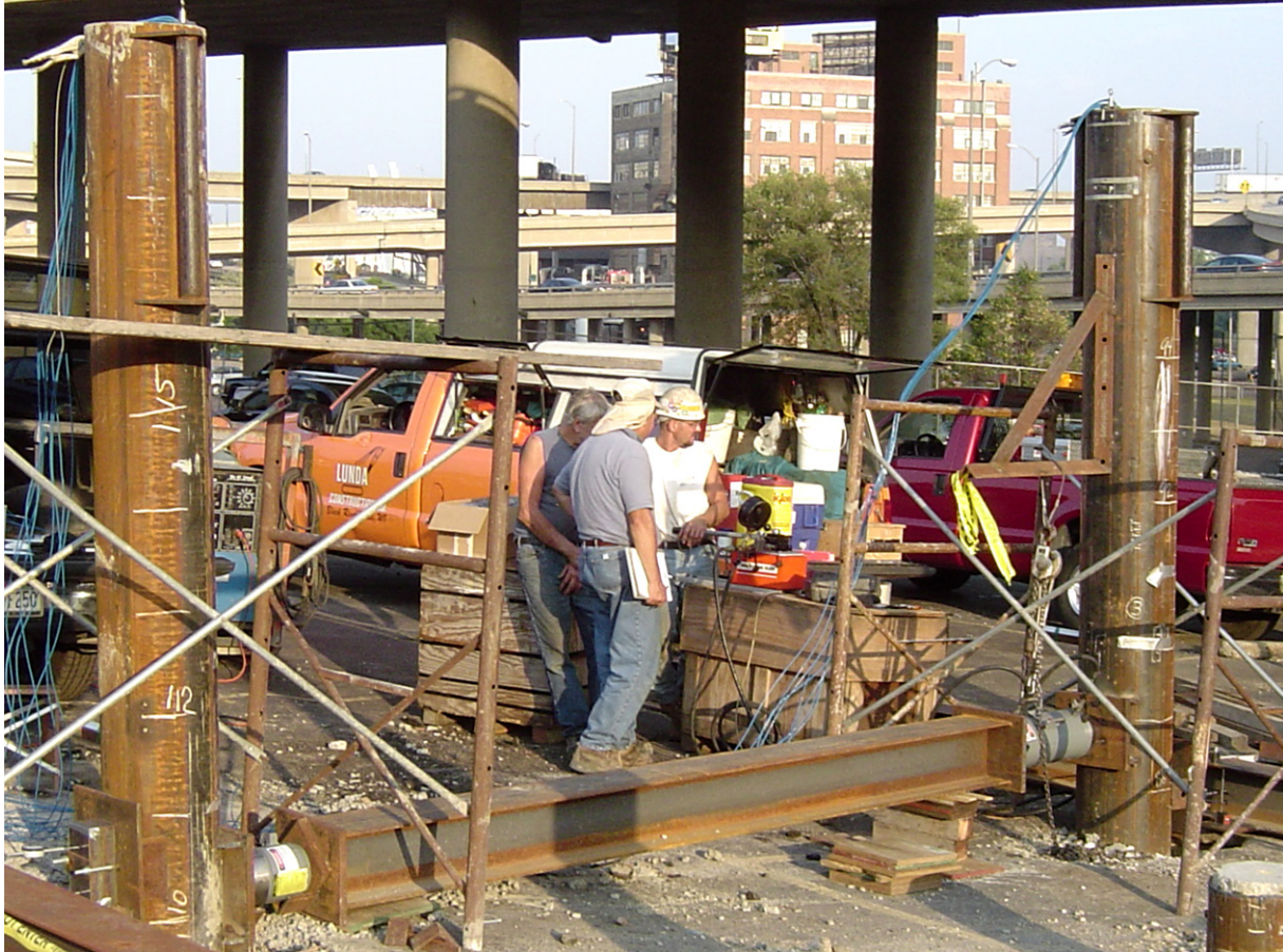
Figure 9-12 Lateral load test on 14 inch and 16 inch O.D. concrete filled pipe piles (courtesy of WKG 2 ).
