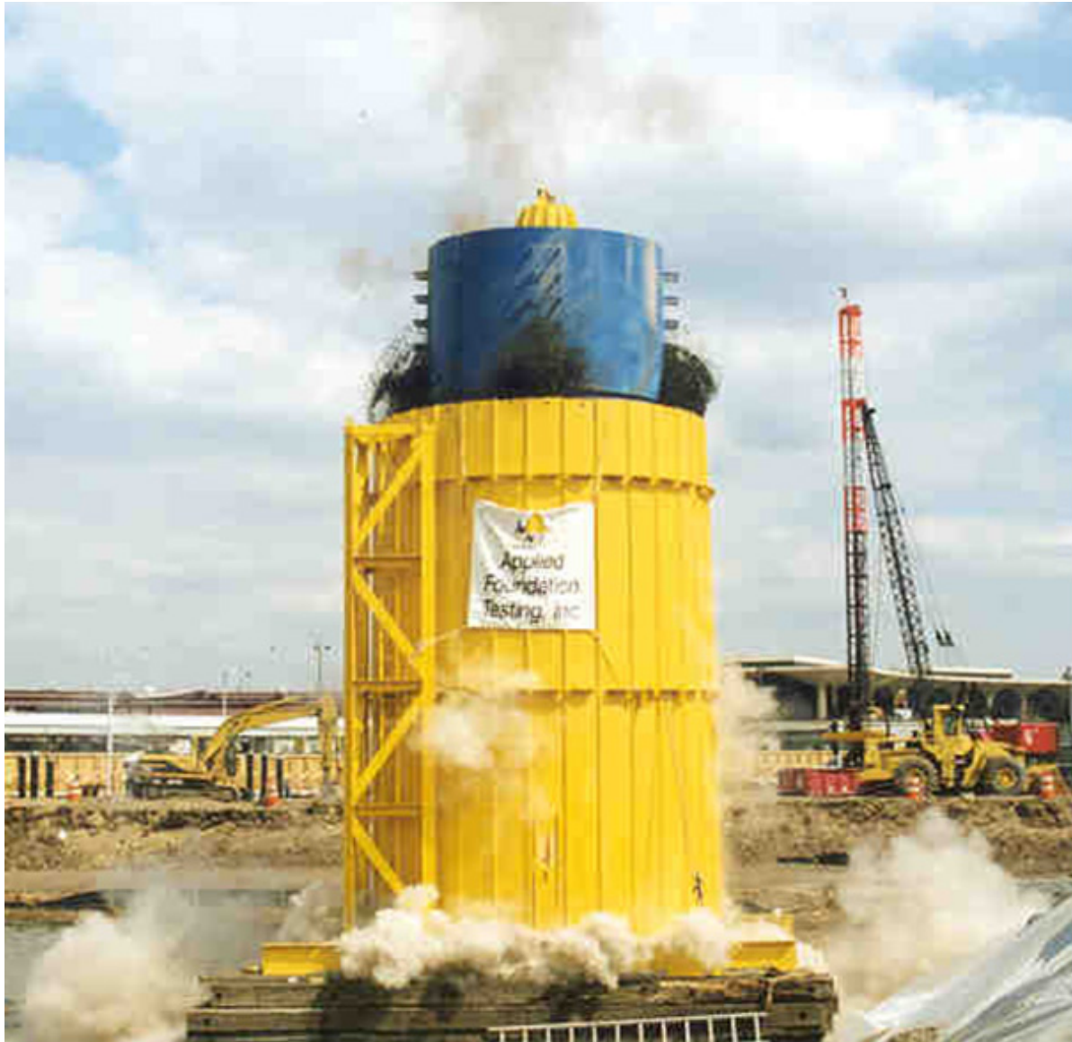
Figure 11-4 Statnamic test in progress with gravel catch mechanism - 9,000 kip device (courtesy of Applied Foundation Testing).
