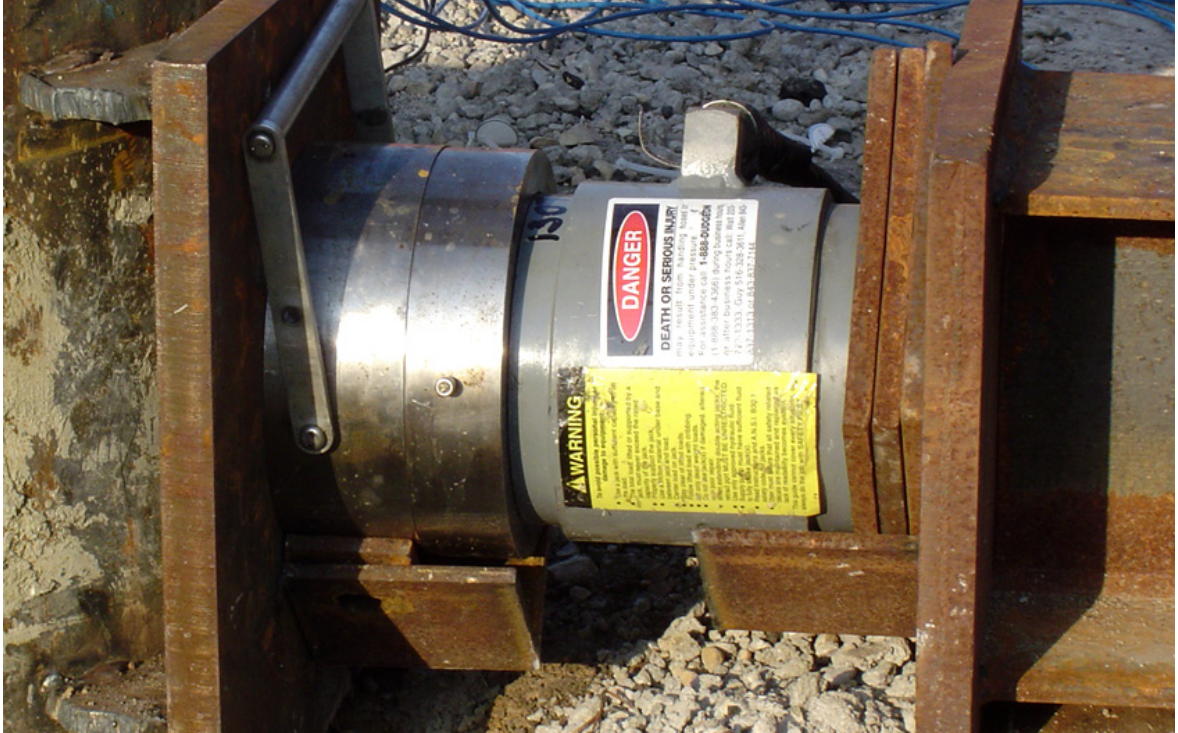
Figure 9-14 Spherical bearing plate and load cell for lateral load test (courtesy of WKG 2 ).
