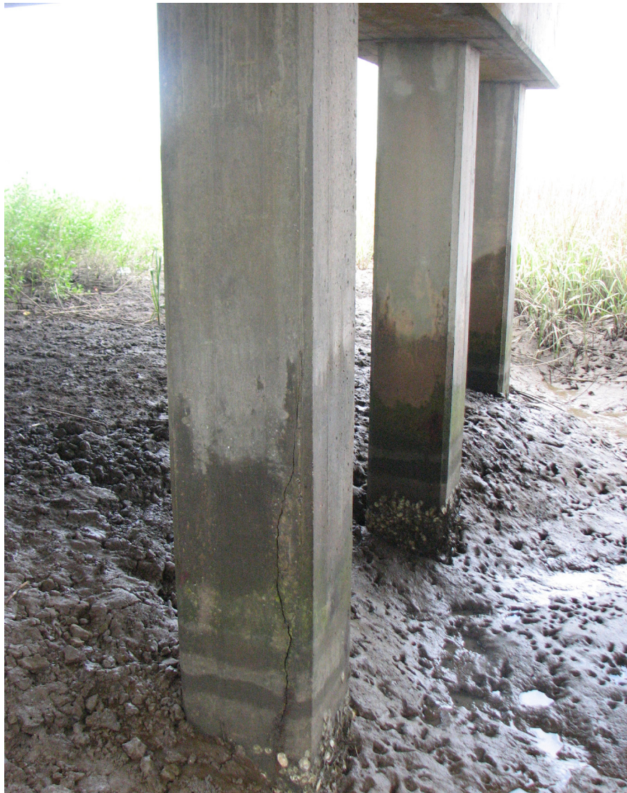
Figure 3-11 Concrete pile damage from corrosion effects on concrete pile reinforcement (courtesy of Moser 2011).
