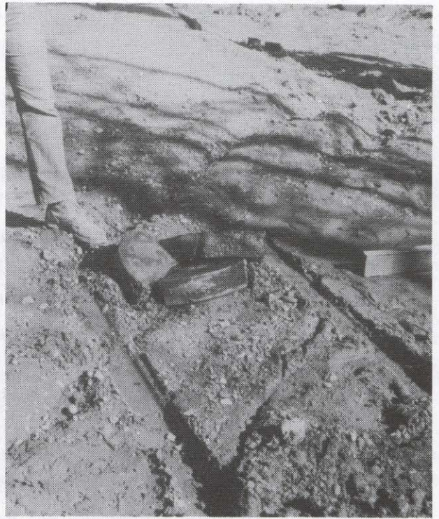
Figure 24.3 Damaged Hammer Cushion
