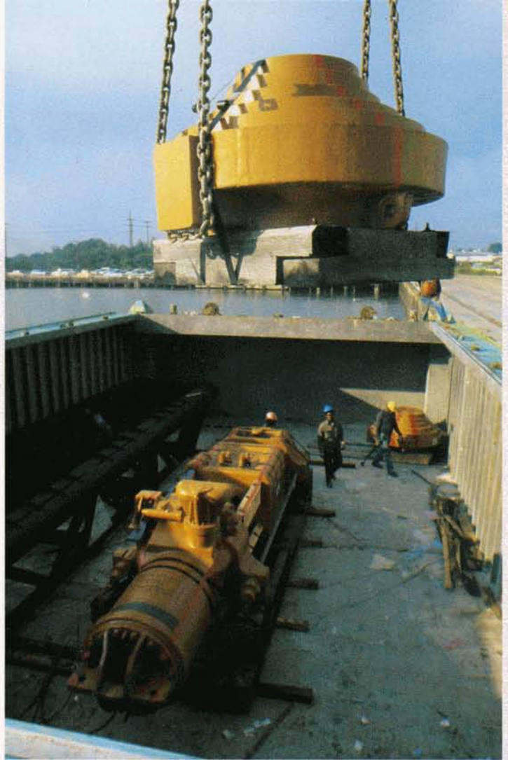
Next, the pile driver cap is lowered into the LASH barge, alongside the hammer section.
