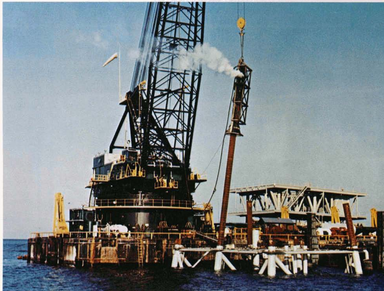
In operation, Vulcan hammer drives pile through leg of off-shore platform, securing it to the ocean floor.
